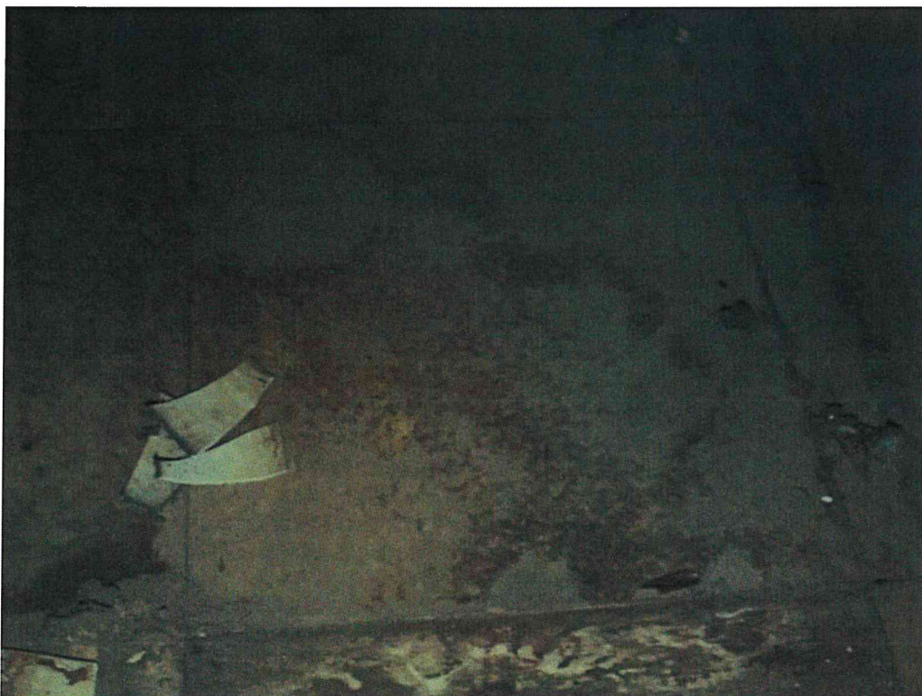
Photo 6 View of HA-9: ACM 12"x12" floor tile with non ACM yellow mastic in HVAC closet.
